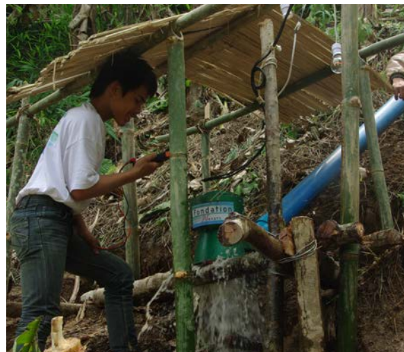
Measurements of the pico-turbine's implementation
