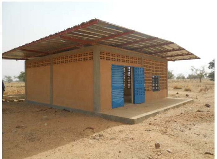
The generator building in Foubé
